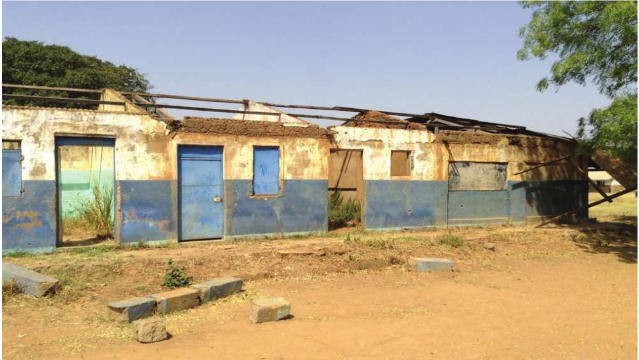
Figure 6: Akworo Primary School classroom block and staff room roof blown off by storm.
